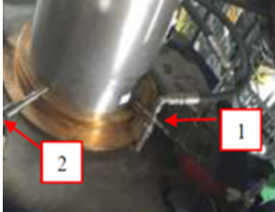
Figure 38: Relative Vibration Sensors for the Measurement of Vibrations between the Shaft and a Stationary Component (Casing or Bearing Housing)
