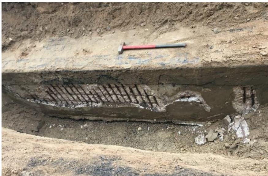
Figure 4. Reinforcement corrosion in concrete walls for concrete culverts, Furutorpsgatan in Helsingborg (photo Öresundskraft).
