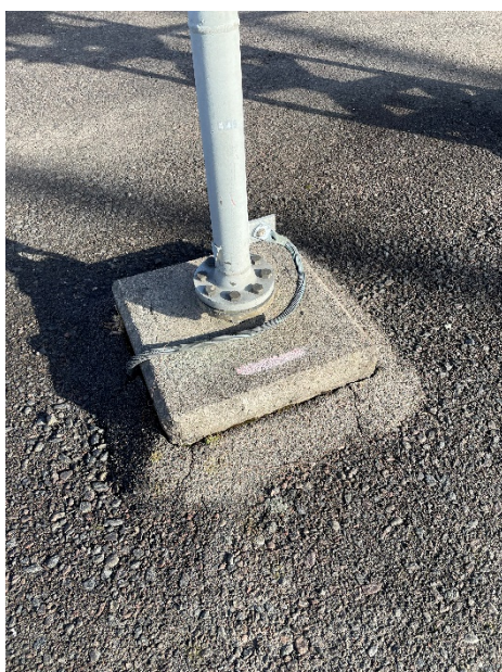
Figure 5 Connection to the earthing grid
