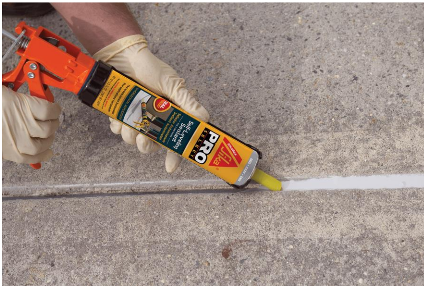
Figure 1. Application of a joint sealant between two concrete blocks. Picture was taken from [1].
