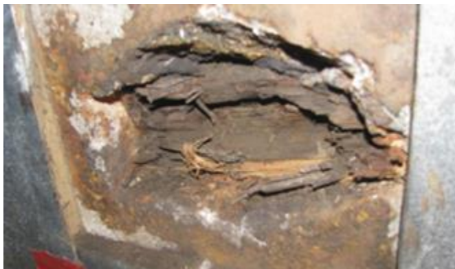
Confinement liner corrosion, Operating experiences summary, Technical letter report - revision 1, Darrell S. Dunn, April L. Pulvirenti, and Matthew A. Hiser U.S. Nuclear Regulatory Commission Office of Nuclear Regulatory Research.
