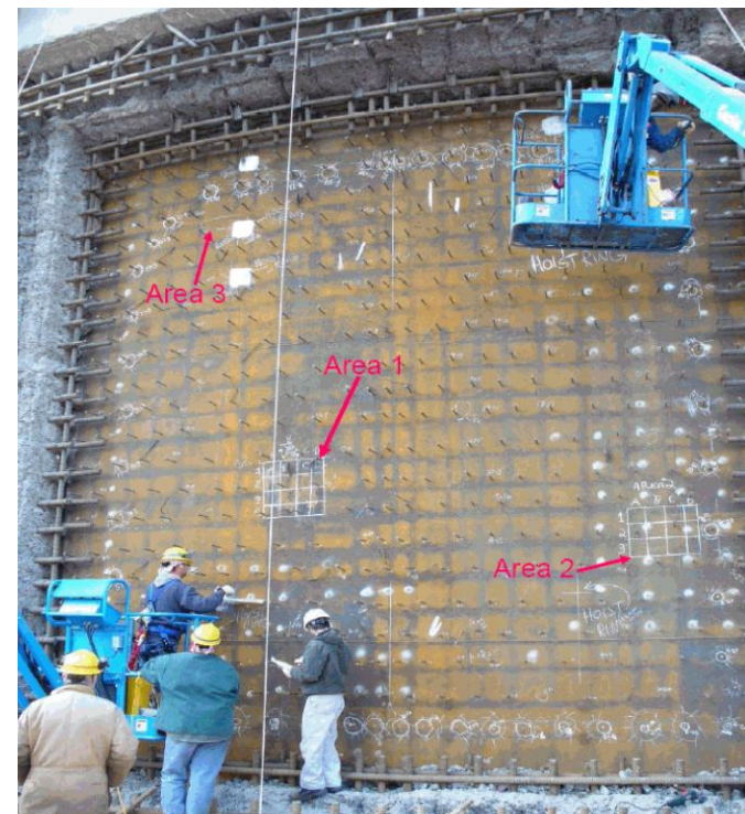
Containment liner corrosion. Operating experiences summary. Technical letter report – revision 1. Darrid S. Dunn, April L. Pulvirent, and Matthew A. Hiser U.S. Nuclear Regulatory Commission Office of Nuclear Regulatory Research.
