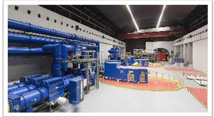
Frades II PSH plant – 780 MW (Portugal) © EDP
