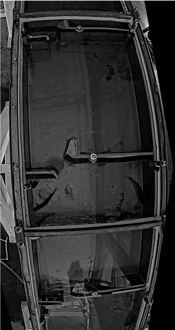
Closed fishway pool 3&4
