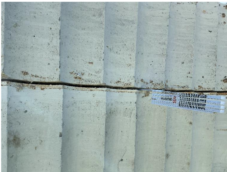
Figure 13. Gap formation observation at Ringhals 2 (2023). (a) Containment wall with the inner wall located on the left side. (b) Containment wall with inner wall located at the top. (Photos provided by Vattenfall).
