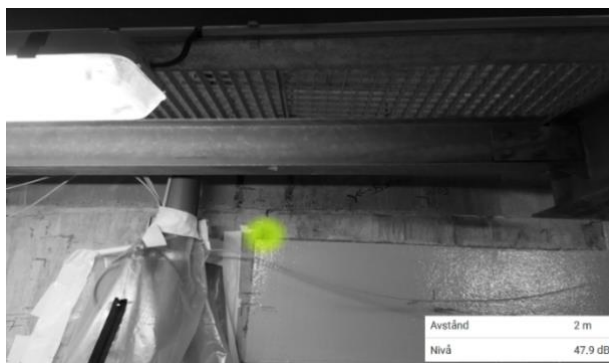
Figure 14 Picture from NL ACOUSTICS of the leakage at reference point 5 – Long distance
