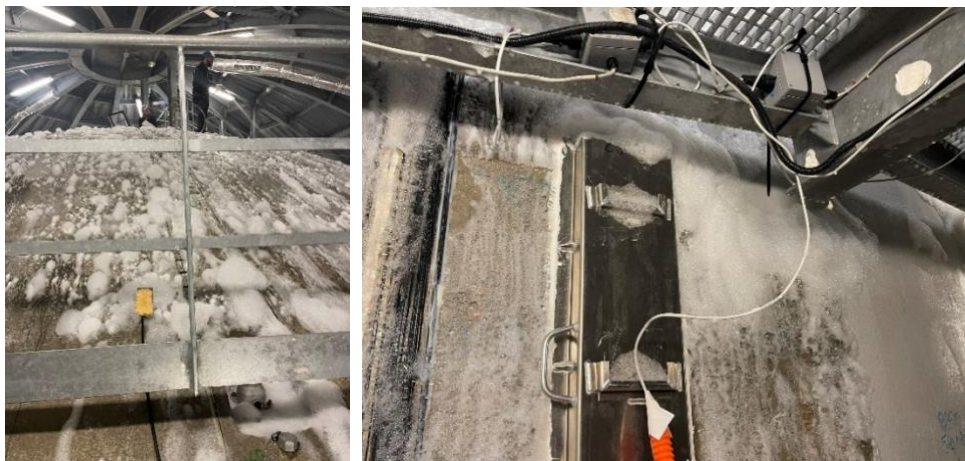
Figure 4 Dome and wall covered by leakage spray
