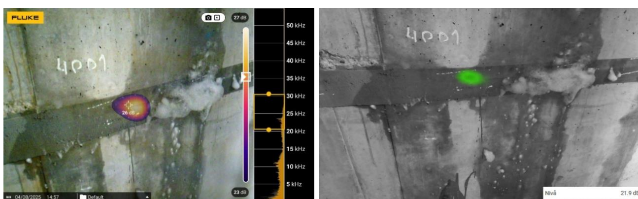
Figure 6 Pictures from the cameras of the leakage at reference point 1. On the left FLUKE ii910 and on the right NL ACOUSTICS
