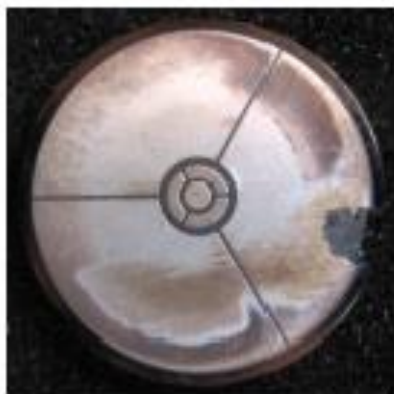
Figure 4-4 Defective thyristor - module SSW1 TH2
